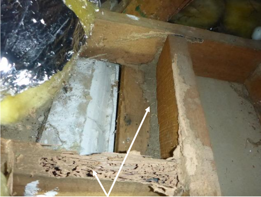
Damaged timber roof frame and termite mud trail in roof
