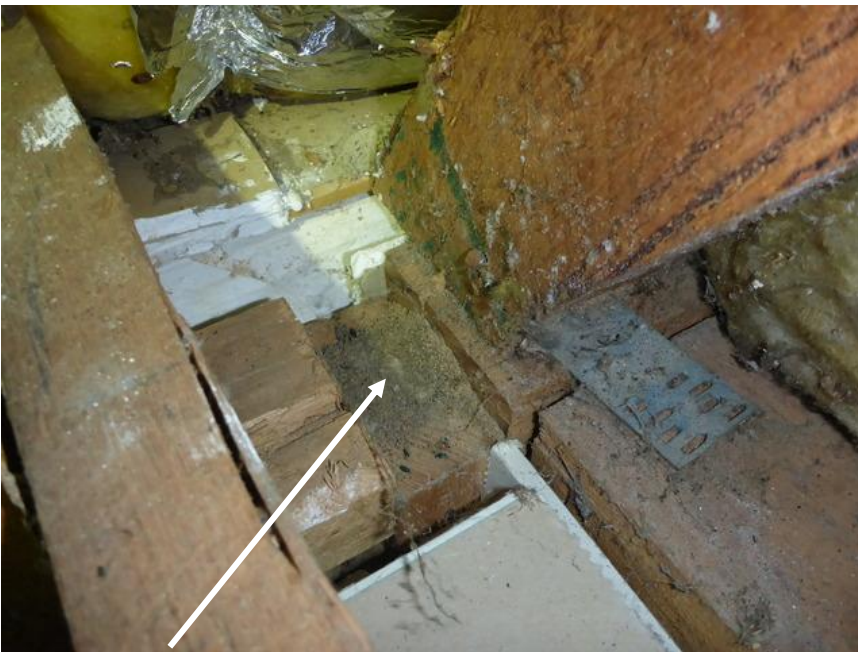
Termite mud trail in roof frame.
