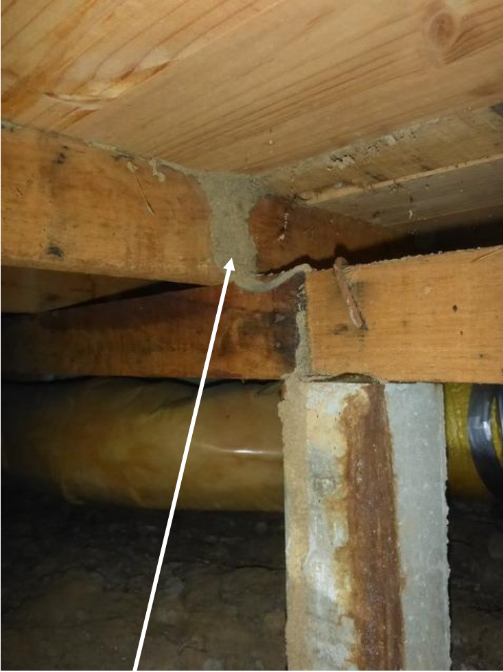
Termites mud trail access to the wall structure.
