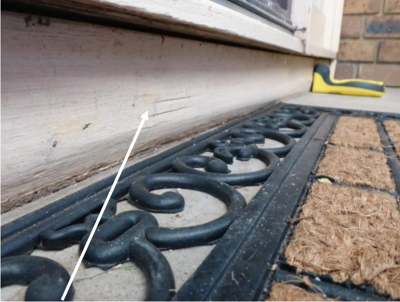
Past termite damage in the timbers under the entrance door.
