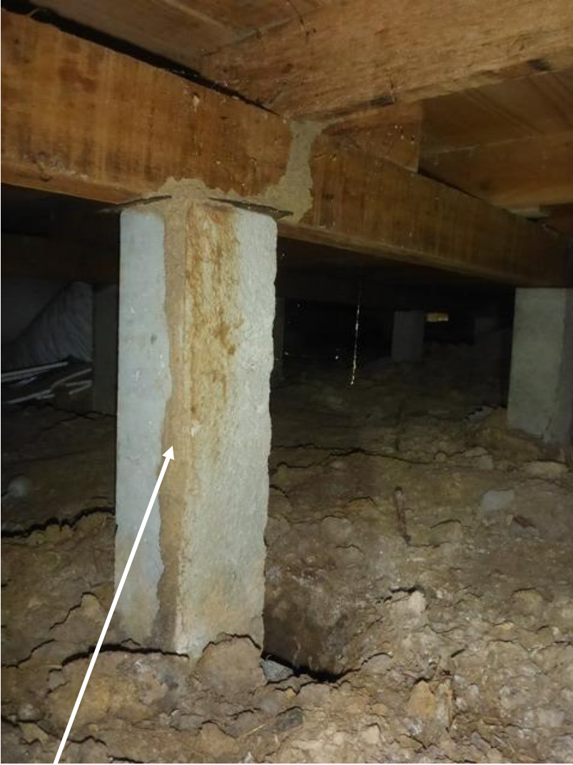
3rd active termite trail at the end of the hallway.
