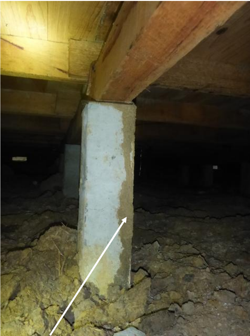
2nd active termite mud trail at the end of the hallway.
