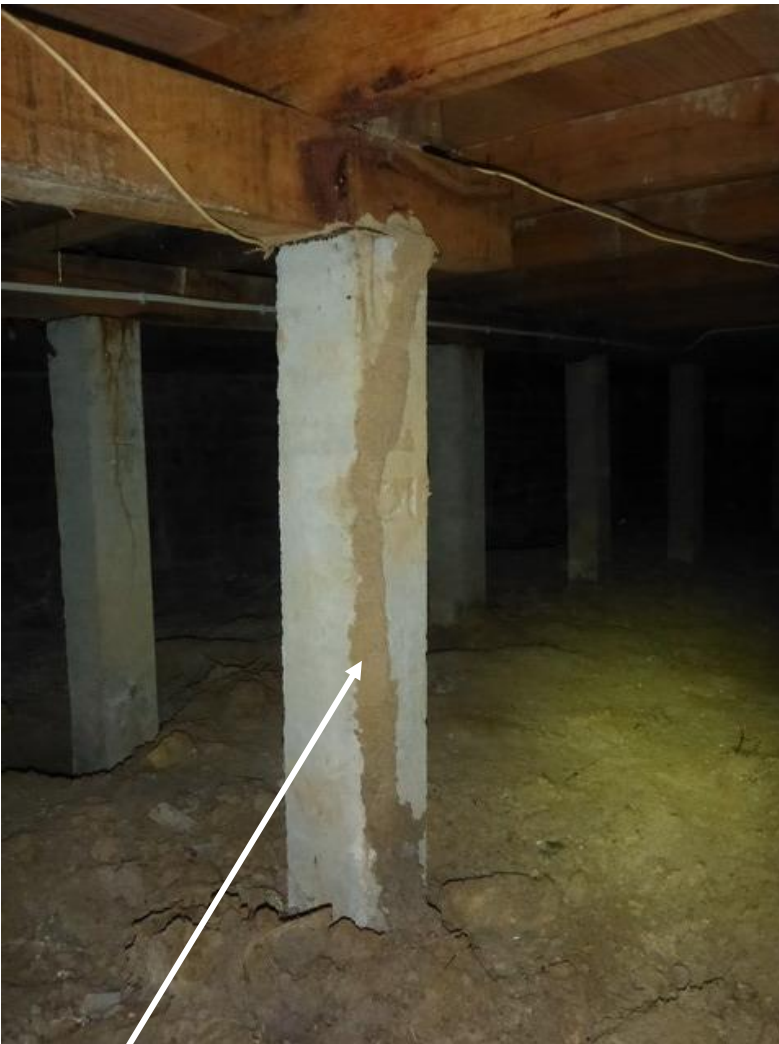
1st active termite trail near the entrance.
