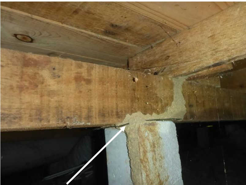
These are substantial mud trails therefore termites have been active for some time.
