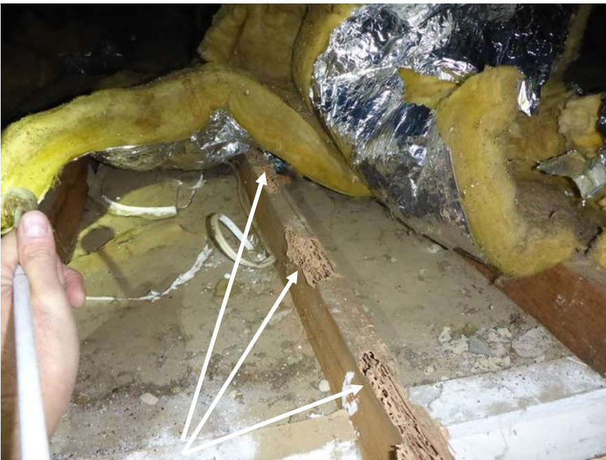
Termite damaged ceiling timbers.
