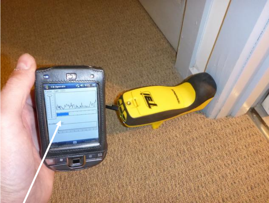
Active termites in the hallway cupboard skirting boards and cupboard door frame.
